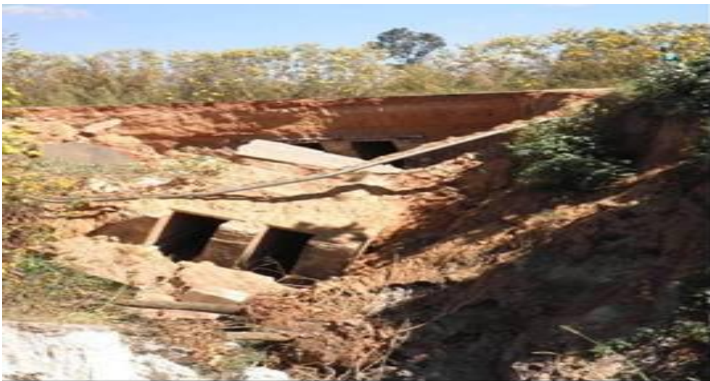
Figure 19: An example of landslide or sinkholes in a sub-urban area
